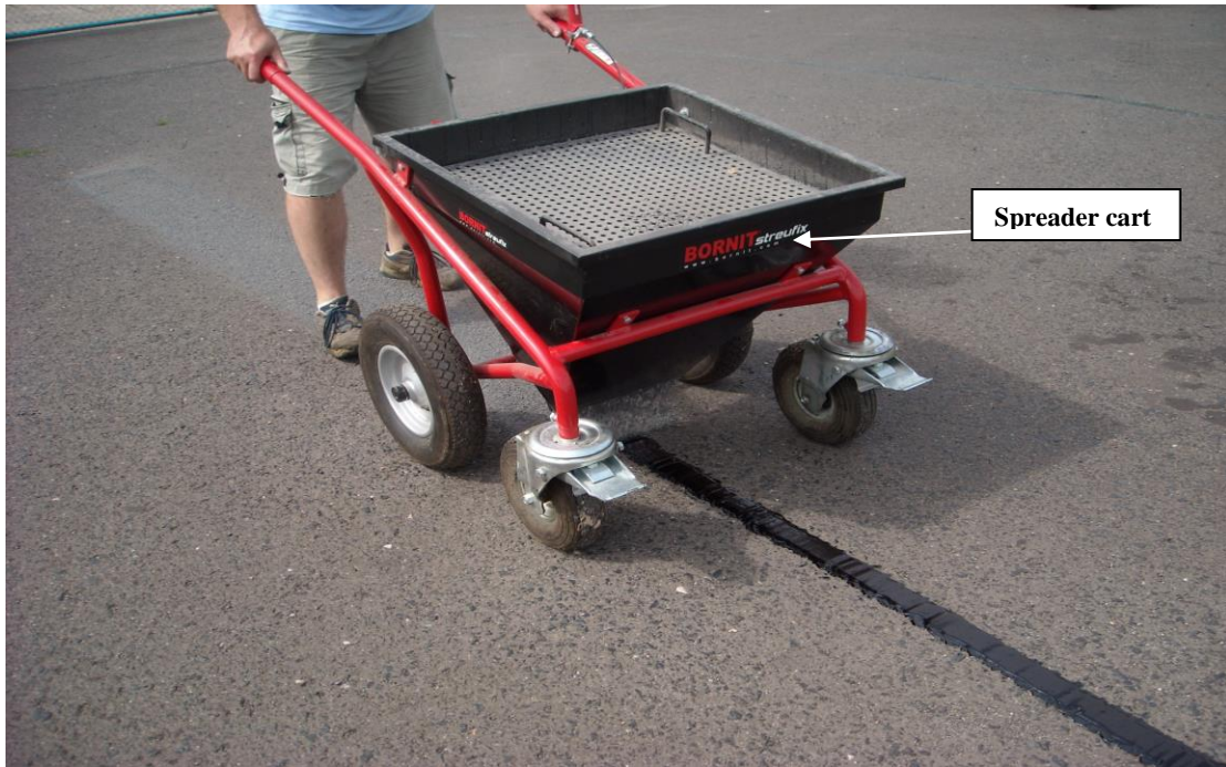
Spreading the treated crack with crushed aggregate of grain size 0 - 4 mm - BORNIT spreader cart
